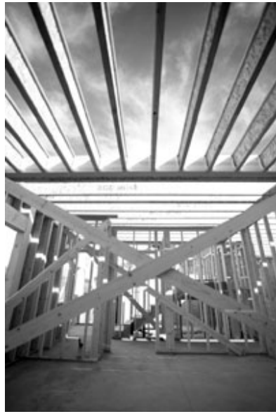
The sky shows through the framing of a house under construction in La Plata County. The Planning Department is undergoing a revision of its current land-use code. Among the things being considered is whether to switch from the labor-intensive "Performance-Based Zoning" to the stricter yet simpler "Euclidean Zoning."/Photo by Stephen Eginore
